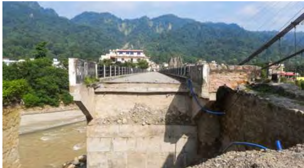
The approach road to the bridge over the Khoh River in Kodtwar was damaged in floods on 8 August 2023
